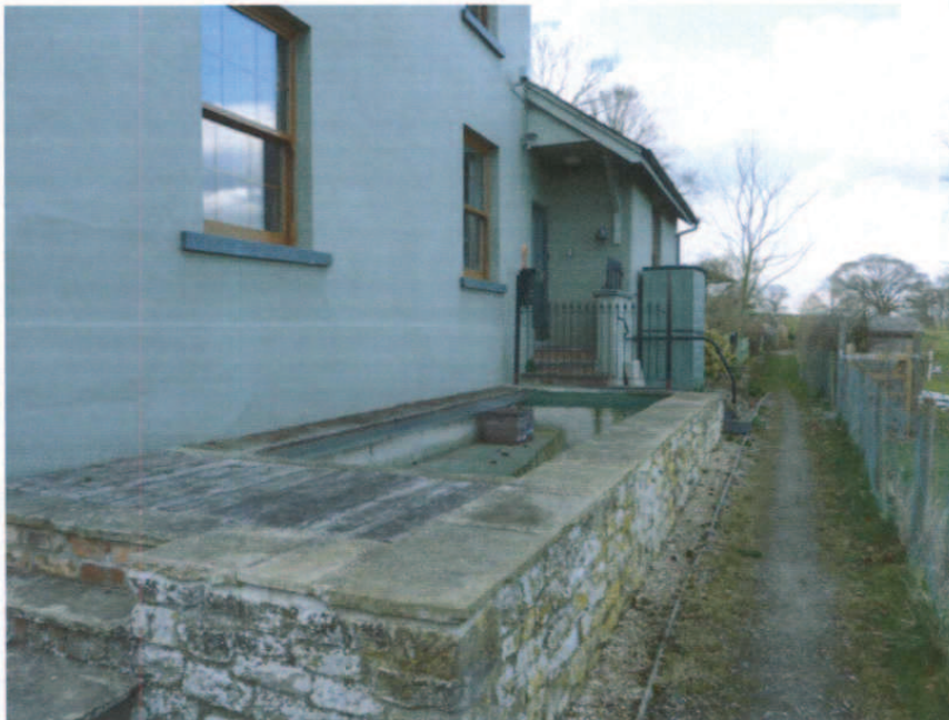
East elevation viewed from private footpath from Water Lane serving Station House and 1-6 Station Cottages
